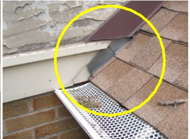
Poor roof flashing- it appears there are no kick out flashings installed. I recommend to hire a licensed contractor to install proper kick out flashings as needed
