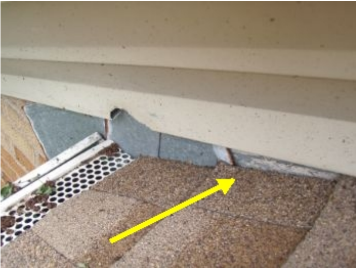
Poor roof flashing- it appears there are no kick out flashings installed. I recommend to hire a licensed contractor to install proper kick out flashings as needed
